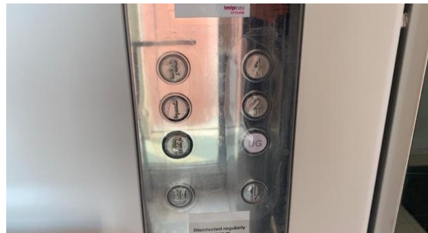
Figure 15. Passenger lift of Tuen Mun Town Plaza (Phase I)
